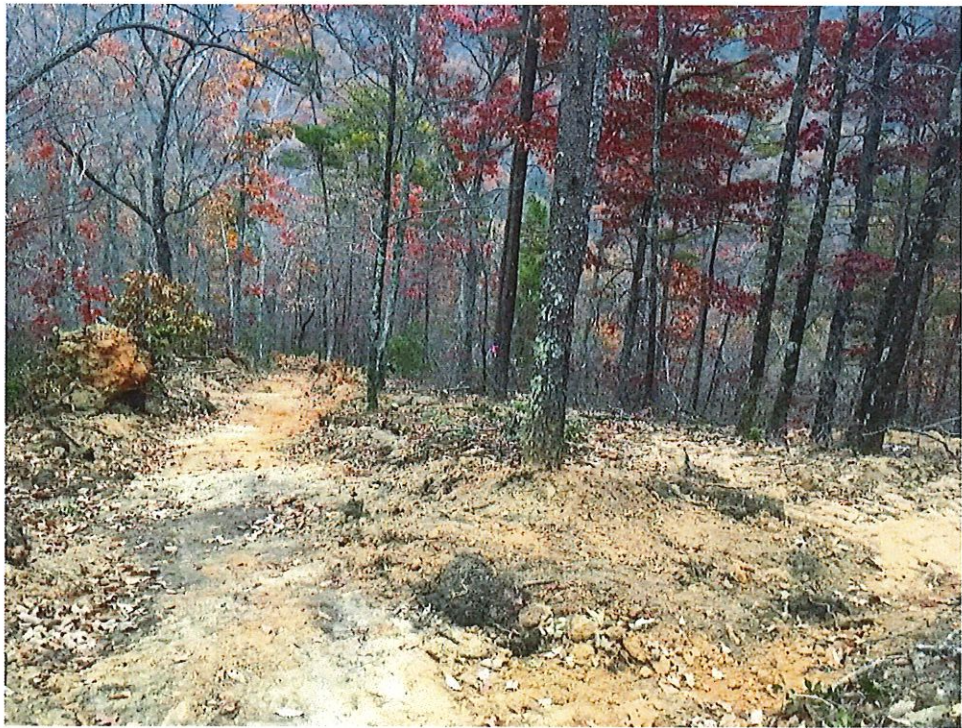
Figure 13. Below grade dozer cut junctions with trail three times, disconnecting turns.
